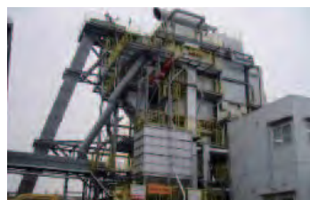
Biomass Boiler (Okayama Plant)
