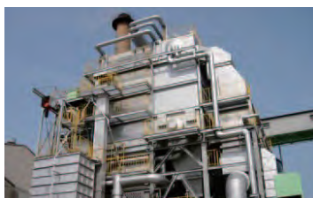
Biomass Boiler (Takahagi Plant)
